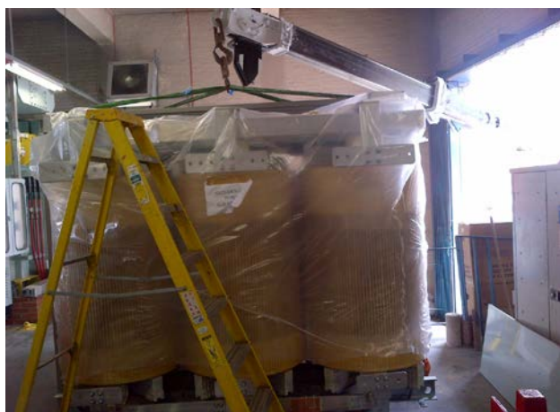
Inverter transformer delivered to Cloudesley Road Substation
